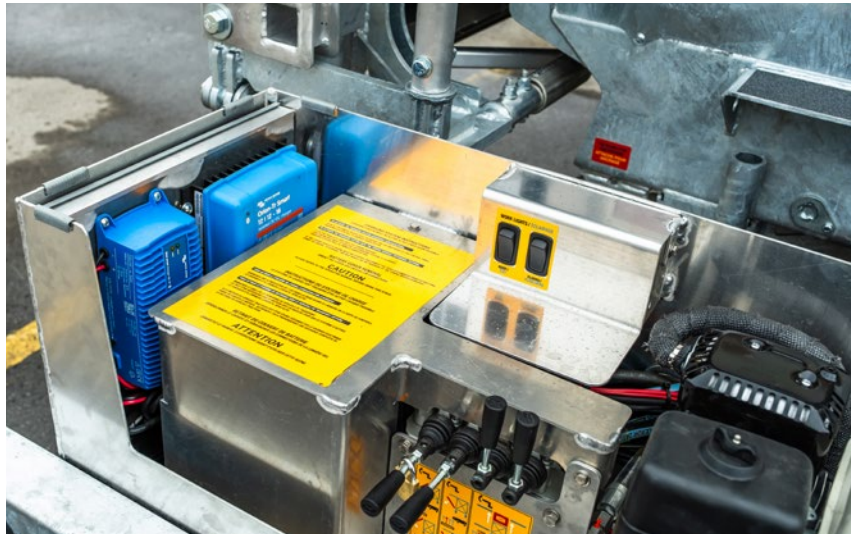
Battery Battery system for work lights, emergency breakaway system and engine starter.
